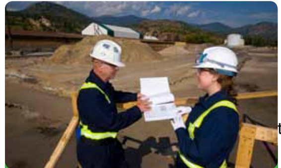
Bill Jankola, Superintendent, Operations Environmental Projects, and Catherine Adair, Community Relations Leader, review plans at the location of a new building under construction to house open mixing and storage of in-process materials, and reduce dust getting into the air.
