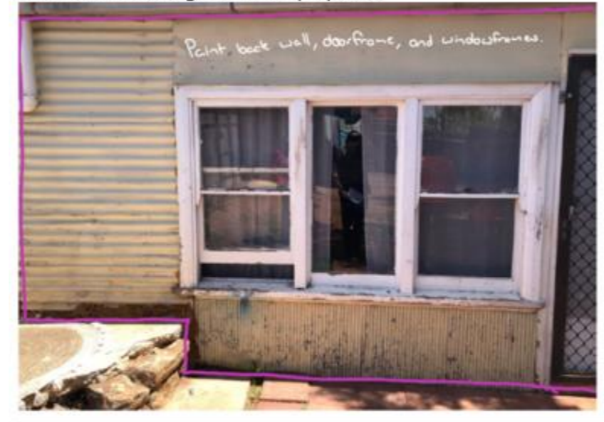
Example 2: Rental. 1 yo, PbB > 10 ug/dL. Blood lead levels rose rapidly after moving into property. Home well sealed internally and internal paint and floors in good condition, but high lead in some soil and very high lead paint (<5%) in very poor condition | on back wall flaking onto child play area.
