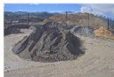
Wind fence to reduce wind speeds that cause dust (Phase 1, 2018, Phase 2, 2025)
